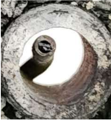
Tip of the water dripping tube obstructed.
