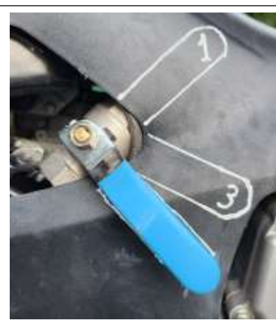
POSITION #2. Completely closed valve.
